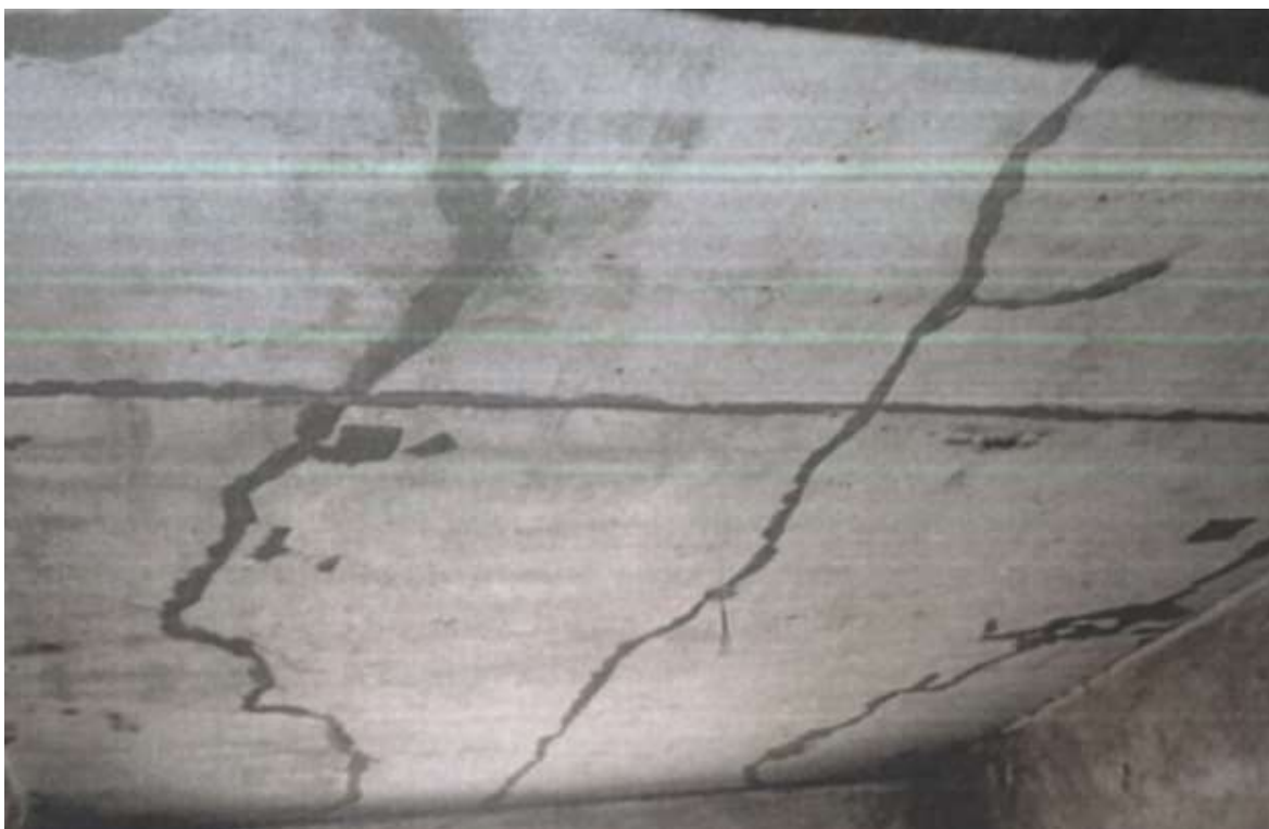
Figure 3.14 - Damage to the ceiling slab of the volume block.
