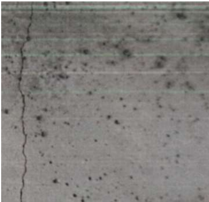
Figure 3.14 - Cracks in the floor (ceiling) slab of the volume block.
